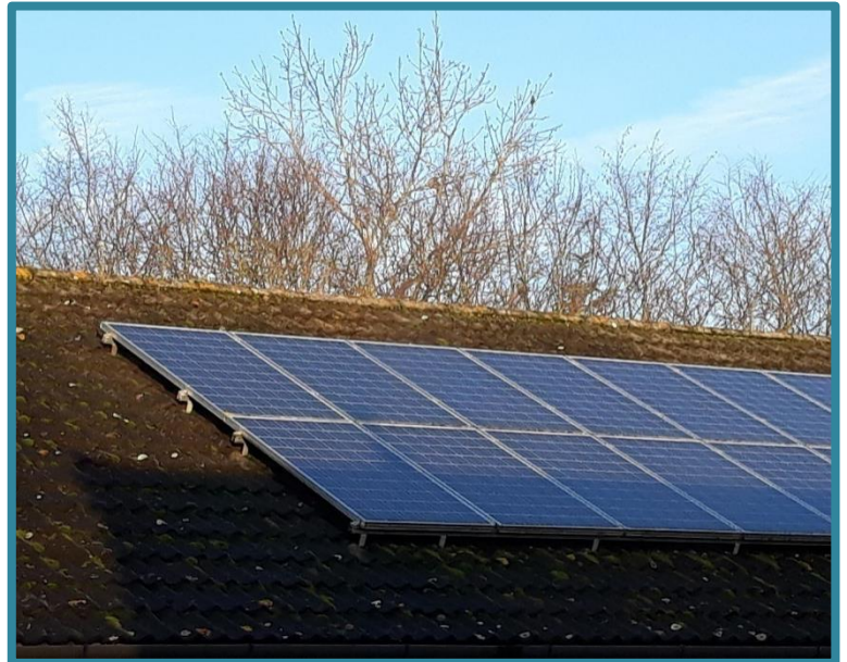
Solar panel shading
